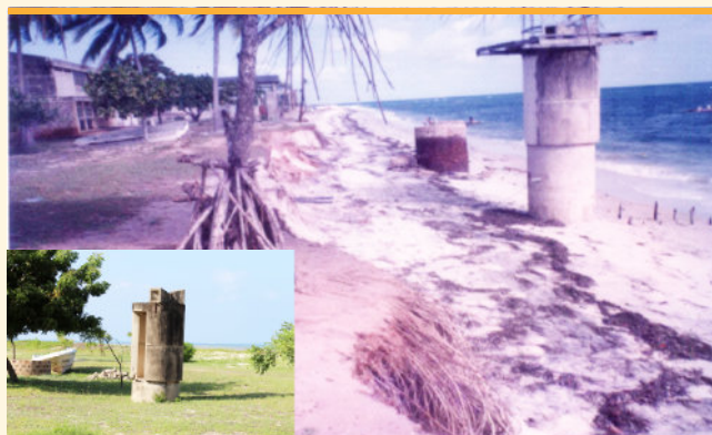
Seawater pumping station and a watchtower of the Kunduchi Marine Biology Station as they appeared being threatened by the beach erosion in December 1995 and current situation (the insert). ©Albogast T. Kamukuru
